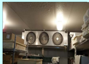
TKS設置後89日経過 (2020/02/26)
